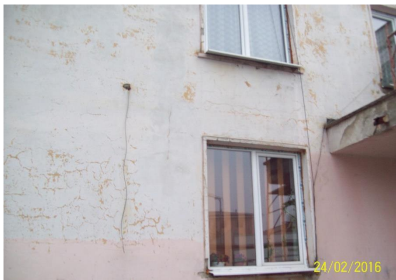
Figure 12 Vulcan Kindergarten - before thermal rehabilitation
