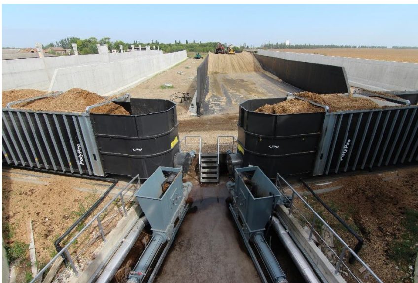
Figure 18 Biogas CHP Plant in Alibunar: Trench silos and biomass feeders of CHP plant
