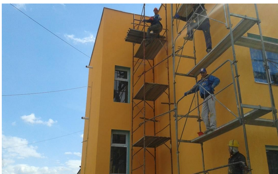
Figure 13 Vulcan Kindergarten - before thermal rehabilitation
