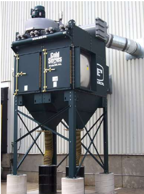
Dust collector at a pastry processing facility.
